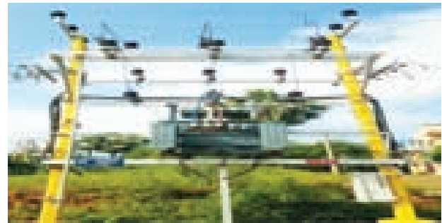
315 KVA Distribution Transformer installed at Dharmapuri in Puducherry region.
