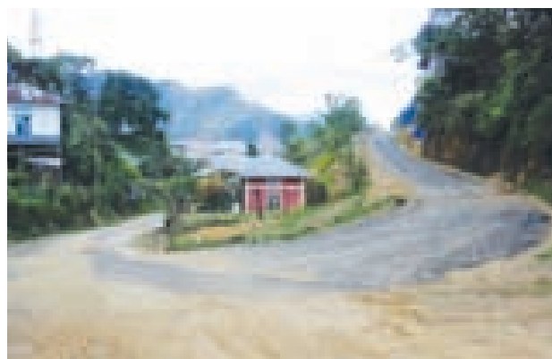
Blacktopping of Internal Road from main Road to Sunday School Hall near 14 th AP
