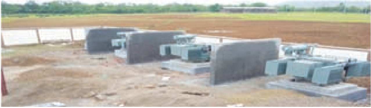
3 MV Solar Power Plant at Velugam
