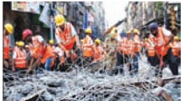
NDRF rescuers during under construction Vivekanand flyover Kolkata, (WB) collapsed
