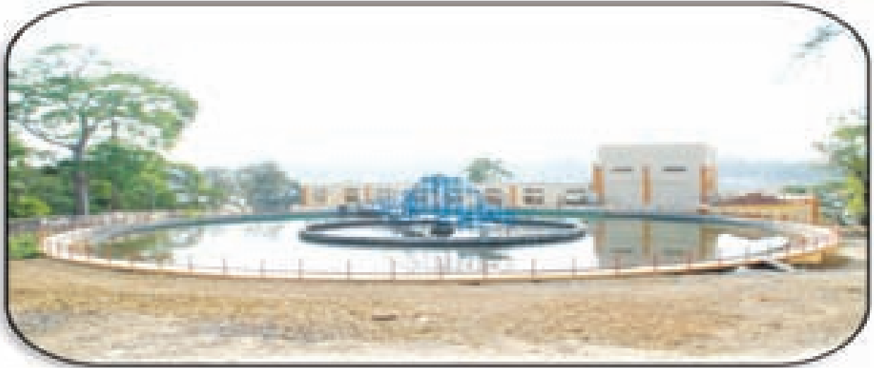
MLD treatment plant at Lambaline
