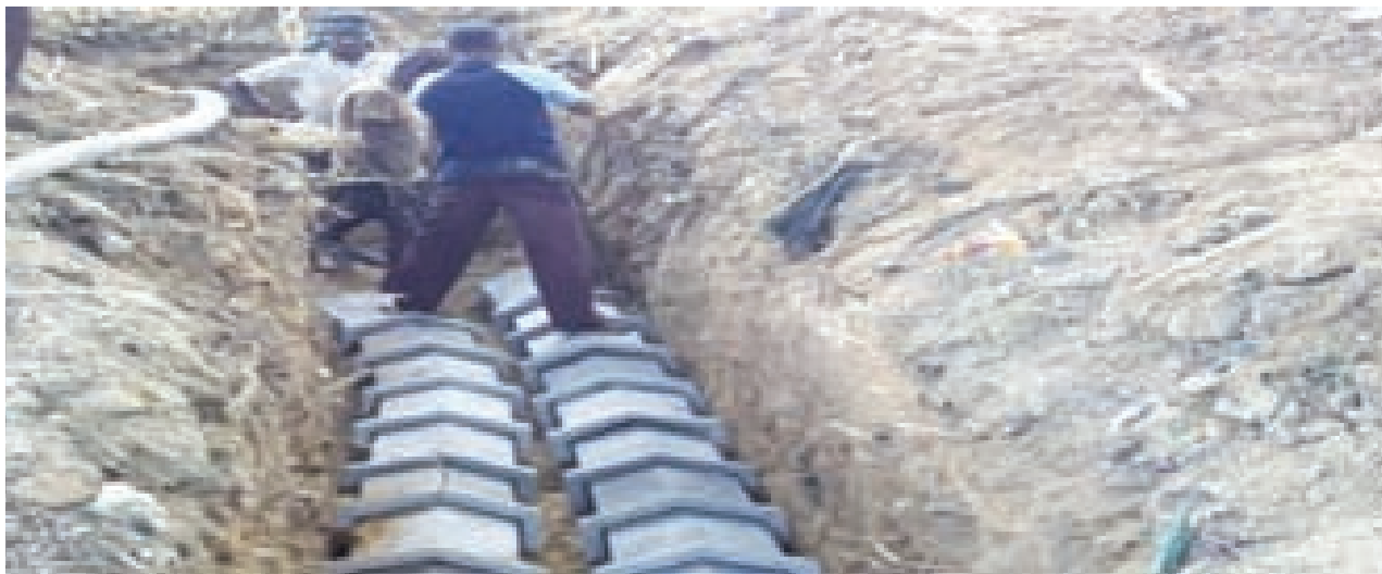
Laying of 11KV Underground cable with protective covering in the trench at Karaikal
