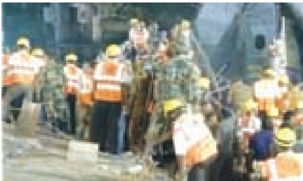
NDRF rescuers during under construction Vivekanand Flyover in Kolkata (West Bengal) collapsed
