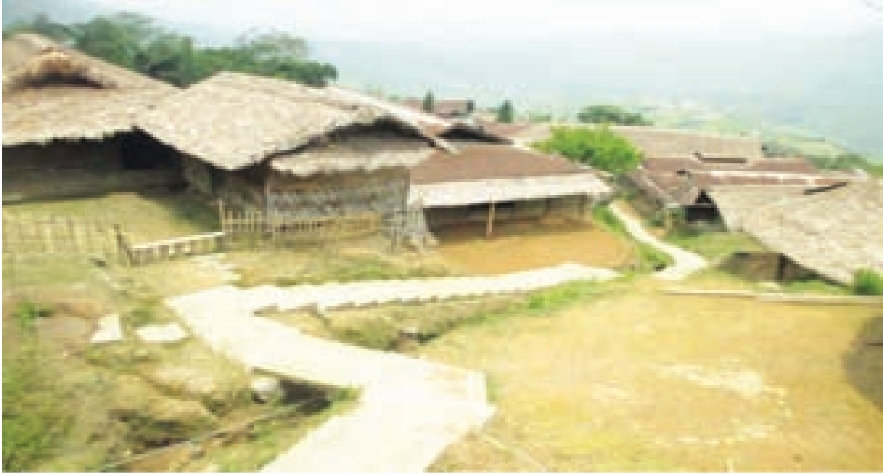
Construction of Footstep at Chingkao Chingha village, (District: Mon) Nagaland under BADP, SCA: 2014-15
