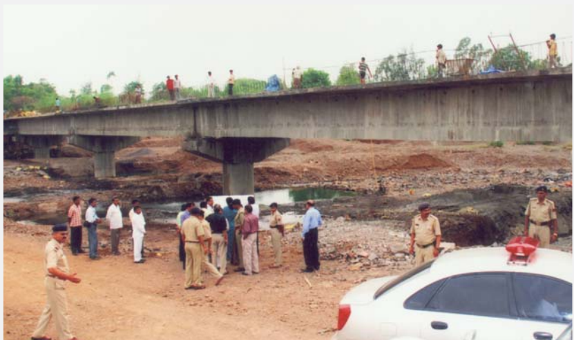
Construction of bridge across rive Sakartod joining Khanvel and Talavali villages, Dadra & Nagar Haveli
